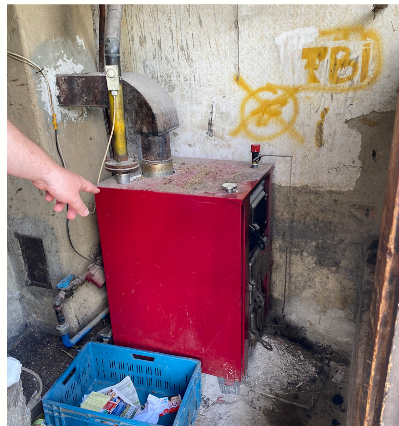
Before: Old boiler (Magyarnándor, Nógrád county)
